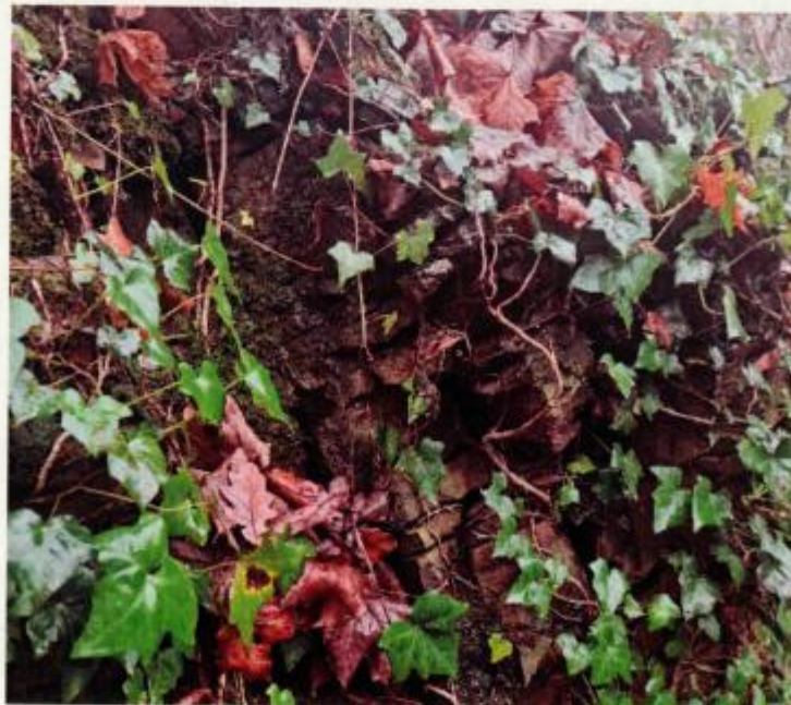
Figure 13: Open close spaced transverse jointing of rock columns at crest of slope
